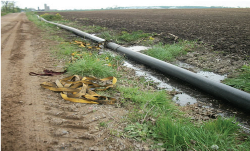
May 1 – SMD dragline breaks along Donnelly Rd. A quick fix with belts does not work.
