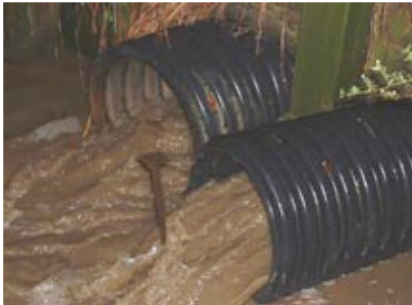
manure discharge, Henning Drain near Hughes Highway, Sept. 20, 2002
