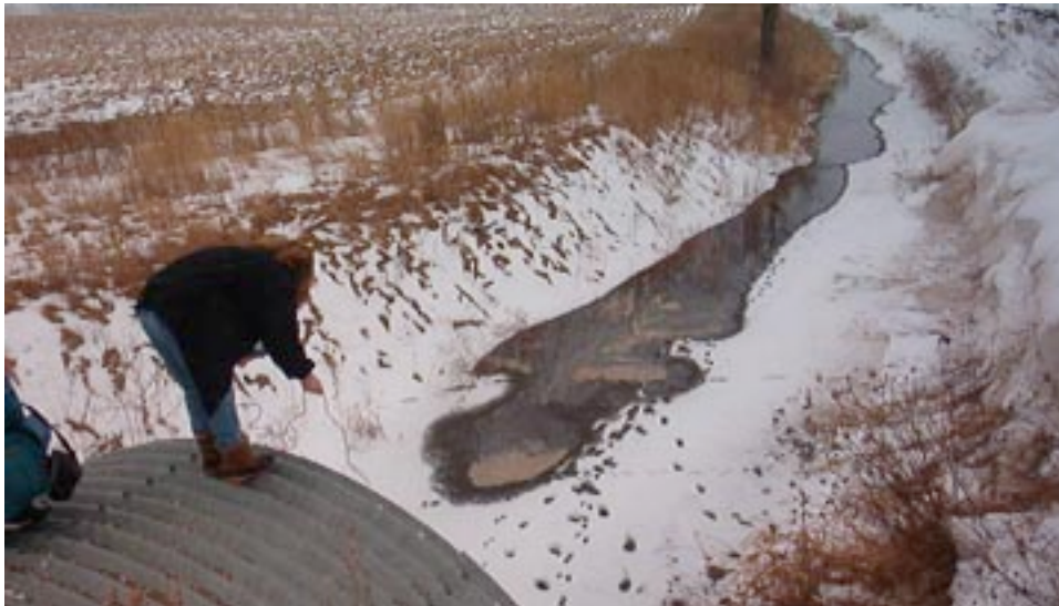
Black manure stream flowing over ice of Toad Creek, approaching culvert at Coman Rd – Jelsma/Mericam discharge (March 2, 2003)
